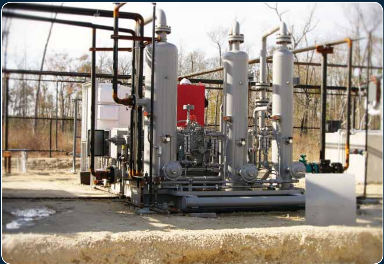
Engineered Concepts packaged this electric compressor as part of an emission free well pad.
