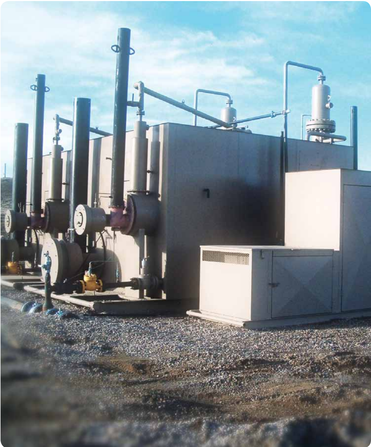
QLD Retrofit Wyoming-Emission free dehydration technologies can be retrofitted into existing systems regardless of the gas content.
